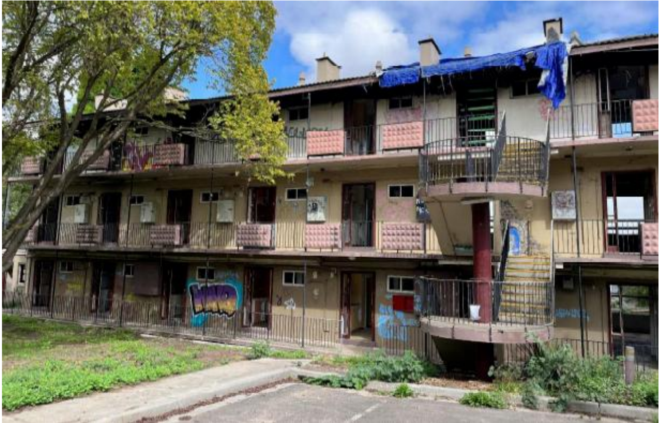
Figure 03 – Recent photograph of 17 Eric Street showing fire damage to the roof
