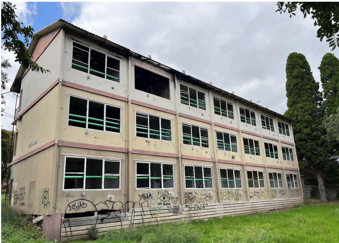
Figure 5 West elevation of 15 Eric Street, showing glazing removed and general dilapidation
