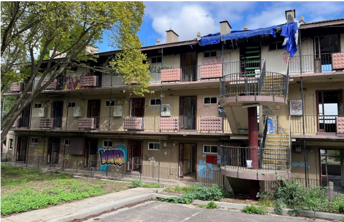
Figure 7 East elevation of 17 Eric Street, note the fire damage to the upper level and roof
